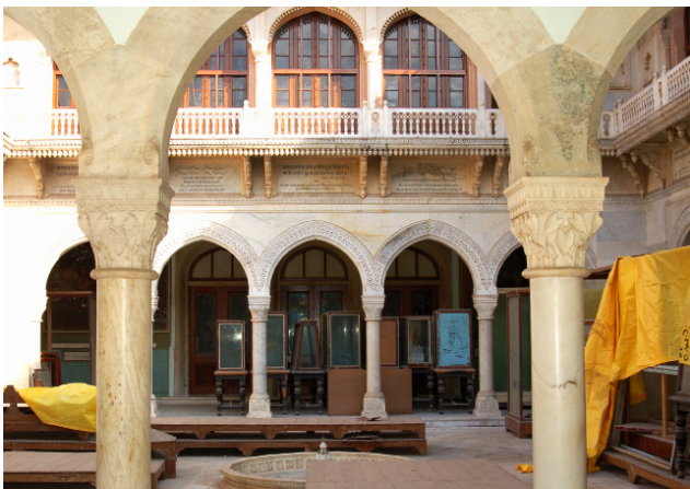
The Jaipur Economic and Industrial Museum (established 1887) under renovation. Photo Sugata Ray
